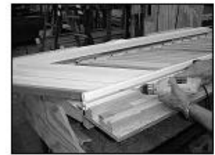
Screw top insert and bottom rail to balusters with 36 2 1/2" galvanized deck screws.
